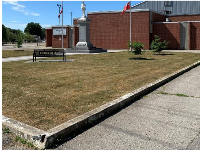
Deteriorated concrete curbs and monuments on the south portion of the site.
