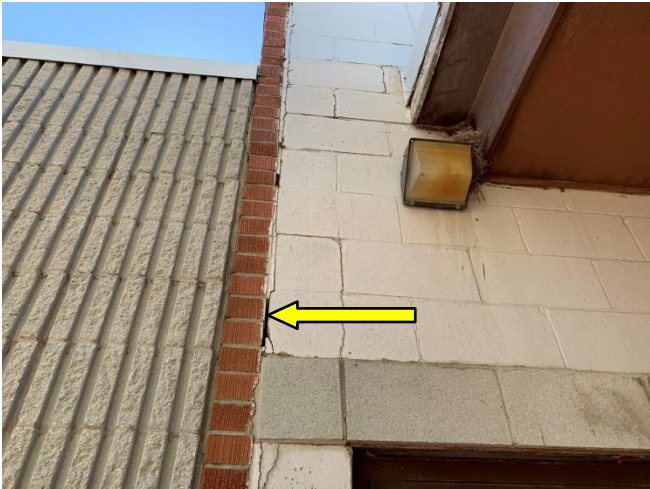
Mortar joint deterioration at the junction brick concrete block masonry.
