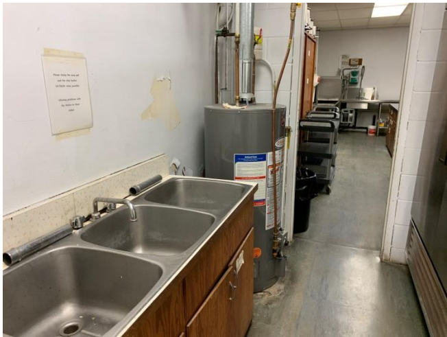
Rental DHW heater tank within the kitchen of the community hall.
