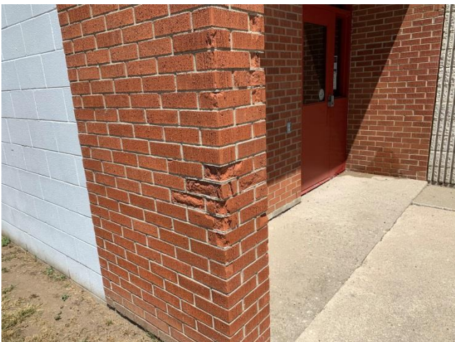
Deteriorated brick masonry units noted on the south elevation.
