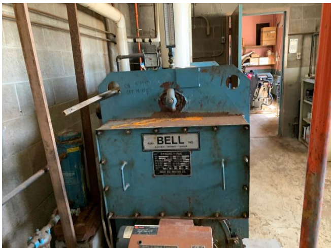
Old heating boiler in the mechanical room.
