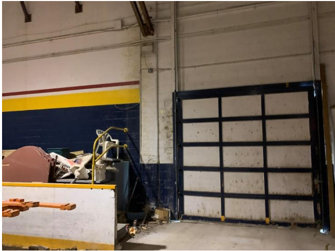
Wood overhead drive-in door on the northwest elevation was noted to be in poor condition.
