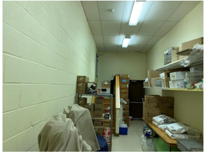
View of typical lighting within a storage room of community hall.
