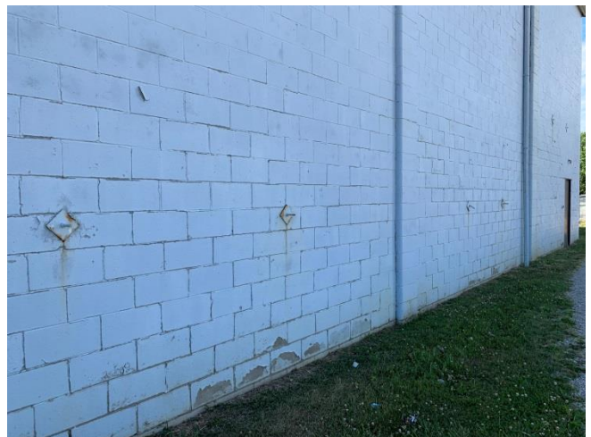
Deteriorated concrete blocks and mortar joints noted.
