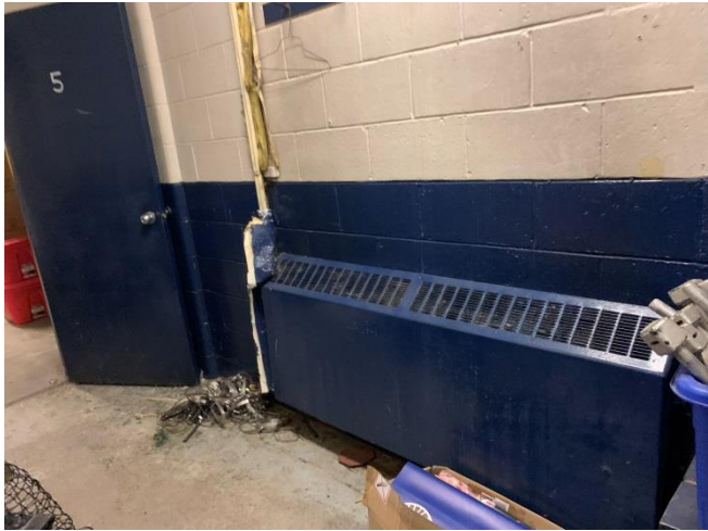
Typical hydronic radiator within a corridor within a room of the central portion of the building.
