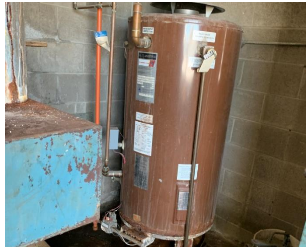
Old DHW heater tank within the boiler room.
