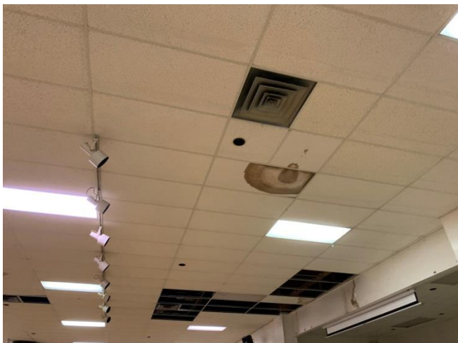
Leak staining noted on the ceiling beneath the BUR system.
