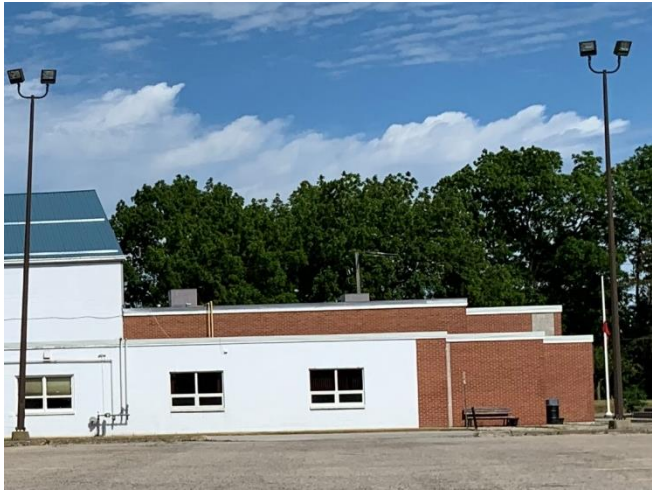
Site lighting standards on the east portion of the site.
