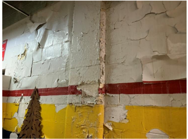
Deteriorated paint on the interior walls of a locker room.
