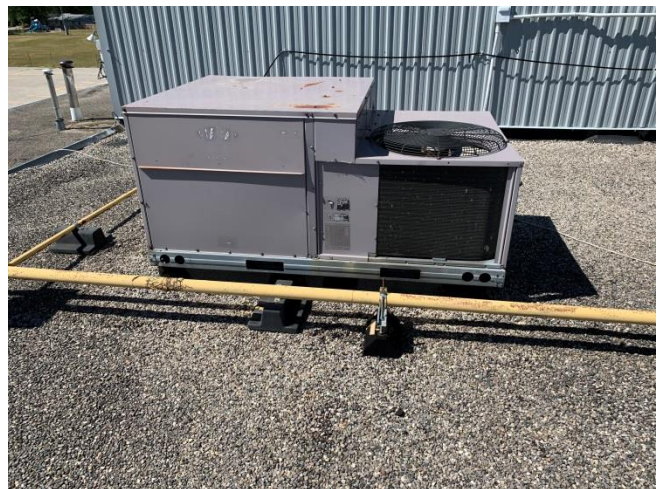
Typical rooftop HVAC unit atop the east roof.
