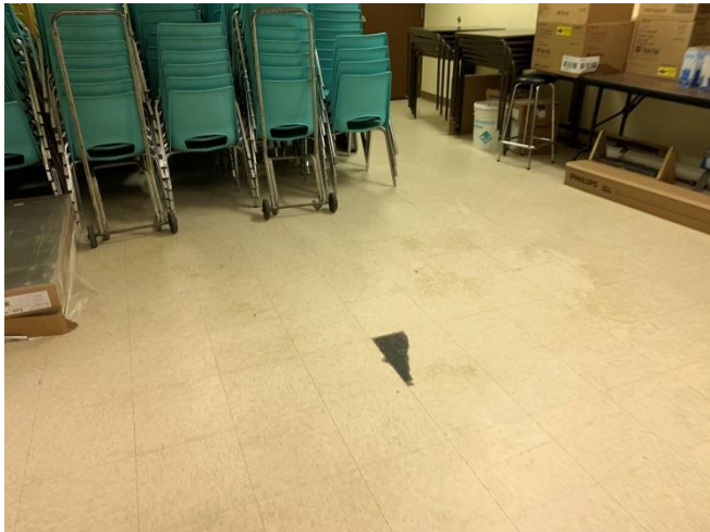
Damaged flooring within a storage room on the south portion of the building.
