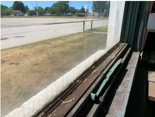
Interior view of a deteriorated window of the building.
